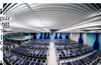
The main CERN datacenter. The 110,000 processor cores and 10,000 servers hosted in its three rooms run 24/7. Source: CERN
